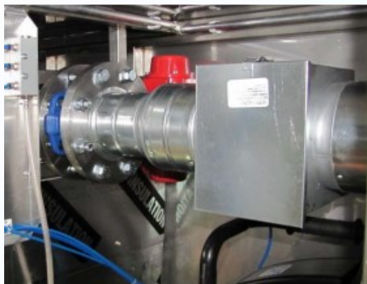
Pictures below: Left and right air inlet pre filters.
