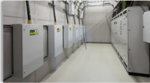
Installed Filter Array
